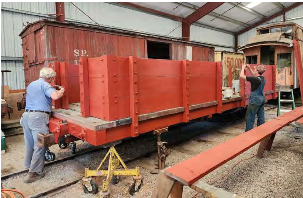
John Stutz is cutting off bolt ends, while David Waterman fits side planks. Photo by AJL Cary
