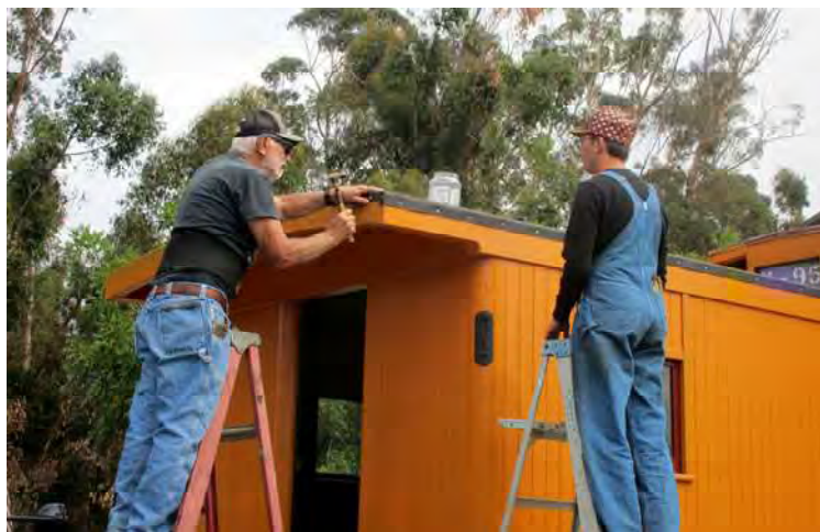
Tony Peters (left) and David Waterman (right) work on the roof of caboose 6101. Photo by Don Marenzi
