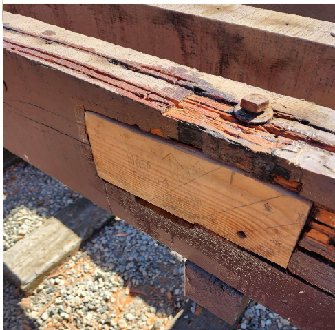
Left: AFTER - The sill now has a wood splice after the crew removed all of the termite damage and termite tunnels.
