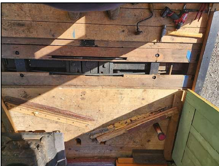
The bolster being decked over showing how the planks have to be relieved for the truss rods (2/13/23). Photo by AJL Cary
