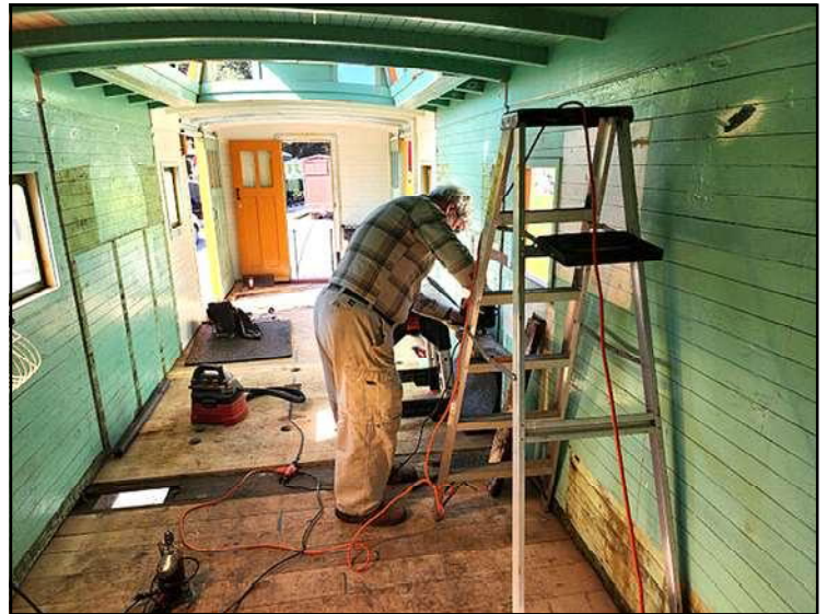
John Stutz trimming a deck plank to fit around a lateral bolster truss rod (2/13/23). Photo by AJL Cary
