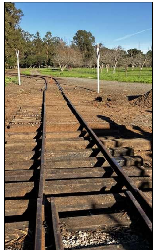
The swing rails will become the stock rails and the 6 new solid ties are in place. (1/22/23).
