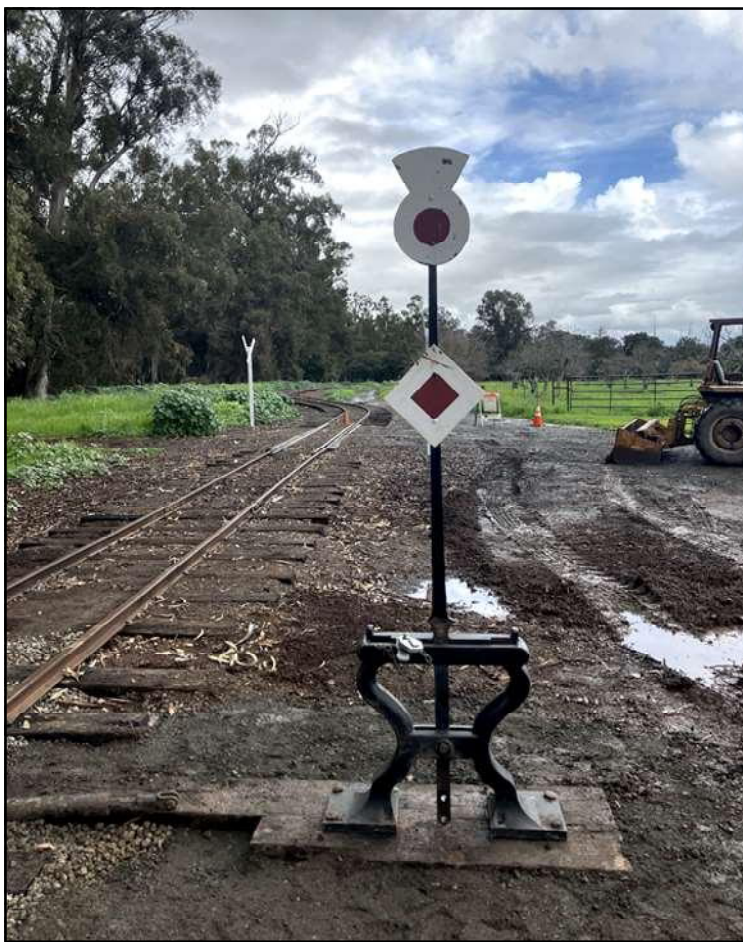
Completed spring switch at Shirley's Siding with Harp switch stand (3/13/23). Photo by David Waterman
