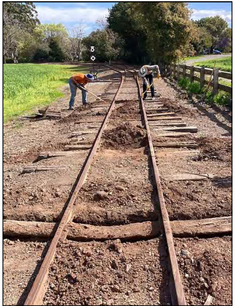
Digging out 39 year old oak ties is a good workout, January-March is the best time to dig for soil conditions.
