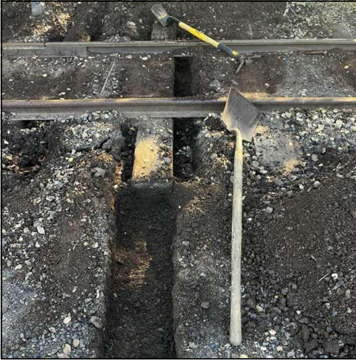
Changing ties in flat ground is tough, we need to dig a slot to slide out the old tie and insert the new tie.
