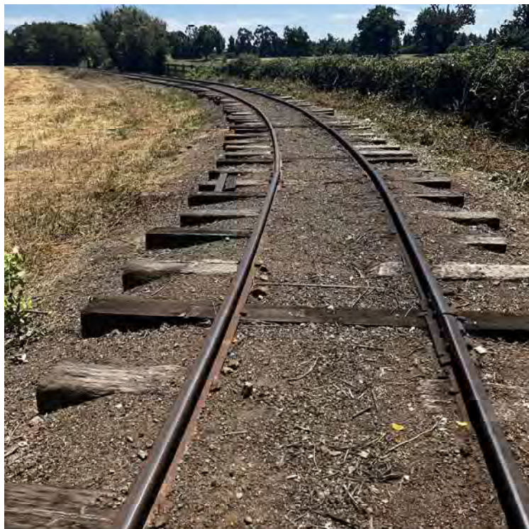
Blackberries gone from roadbed and cut back to fence. Photo by John Goldie
